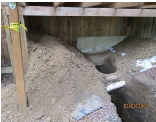
Figure 5. View of work area under deck of house where spoils had been placed at the open edge of the trench
