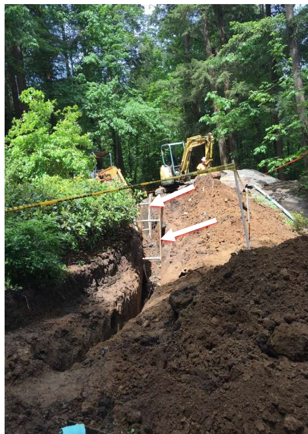
Figure 1. View from front of house: area of incident showing placement of shoring; collapse occurred in between the two pieces of shoring spaced 15 feet apart (indicated by arrows)
